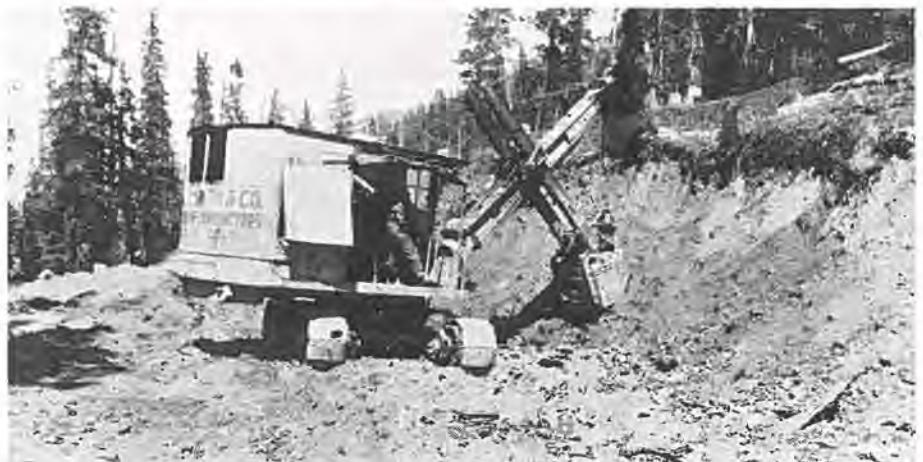
Heavy duty gasoline shovel used by Contractor Luke Smith on new road being constructed by State Highway Department over Loveland Pass.
