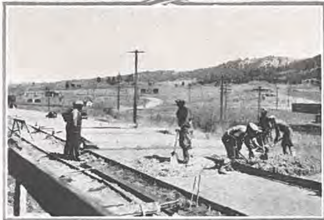
Two views of concrete paving operations near Palmer Lake on the Denver-Colorado Springs highway.
