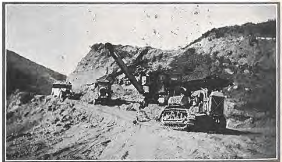
Showing part of the modern equipment employed by the Mountain States Construction Co. in building five miles of new road west of Milner. Photo by A. J. Held.
