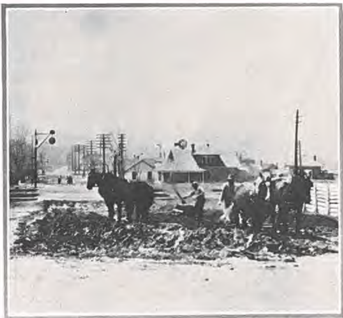
Getting ready for paving concrete section of state highway into the town of Sedalia.
