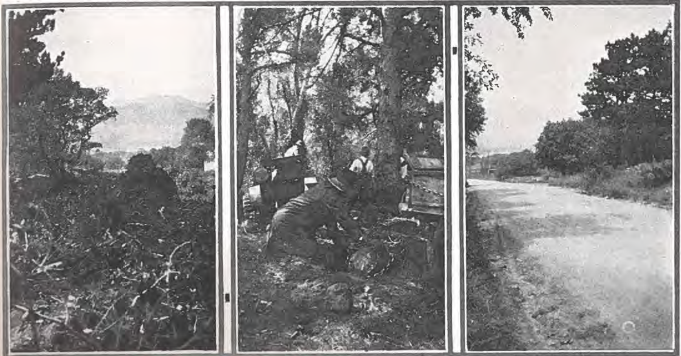
Transformation of new road near Colorado Springs—showing underbrush before clearing, clearing operation and finished highway.
