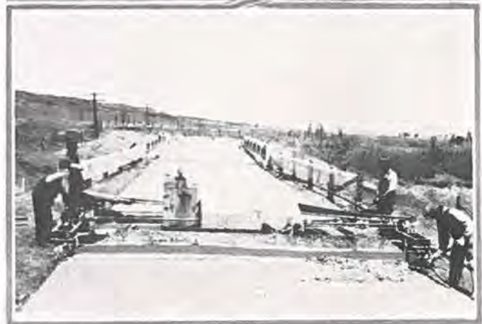
Pouring concrete on the paving project between Tomah and Monument. Lower photo shows finishing machine in operation.
