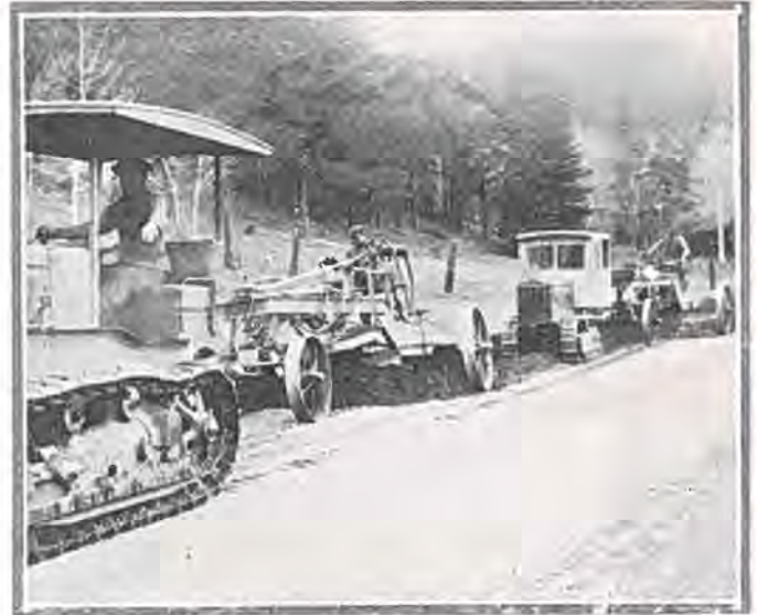
One of Park county's modern motor-grader maintenance outfits. Similar units will be employed by the state in maintaining the 3,300 miles of federal aid roads in Colorado.
