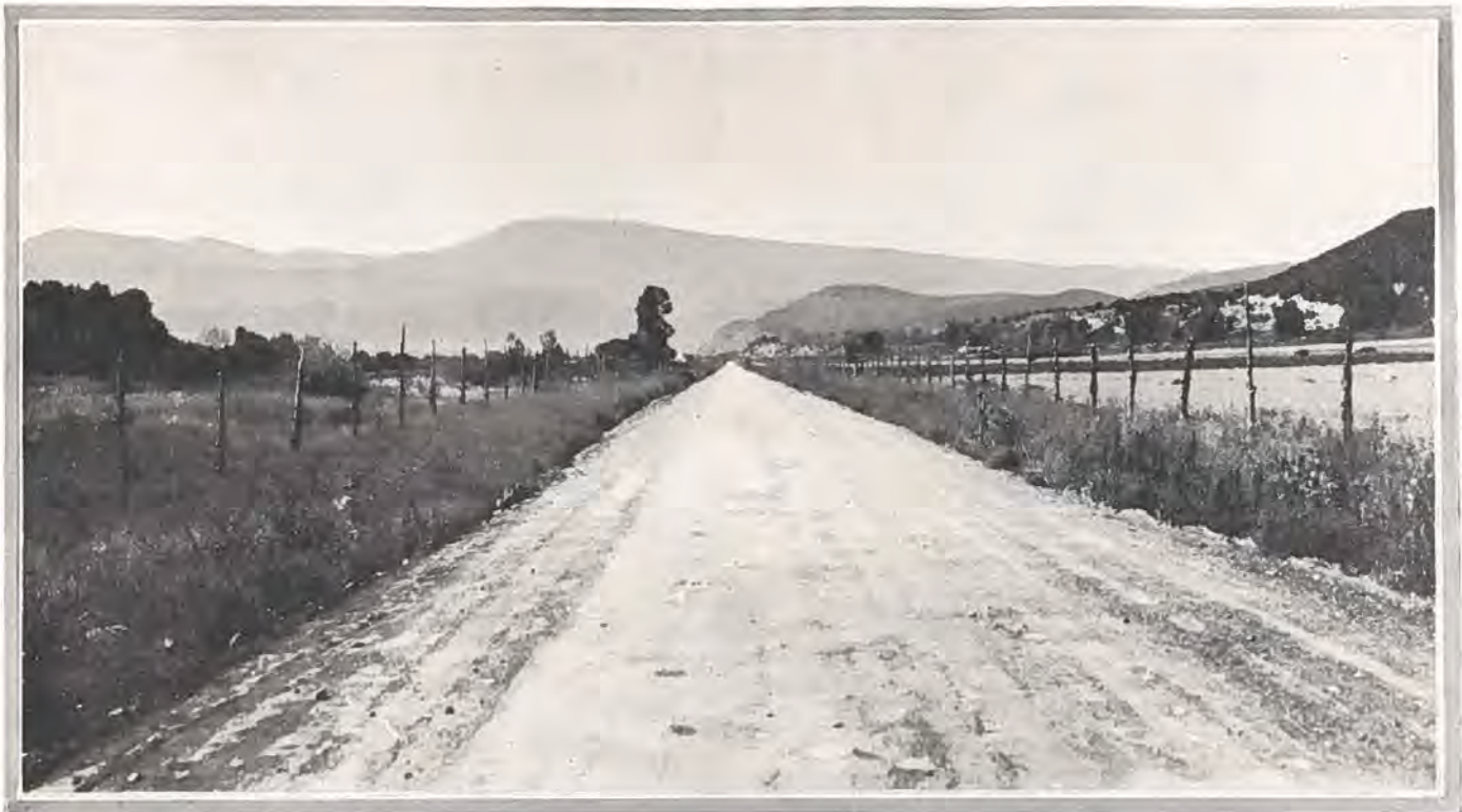
Making an old railroad grade into a high class state highway. This photo shows the reconstruction of the Colorado Midland right of way in Garfield County near Catherine.
