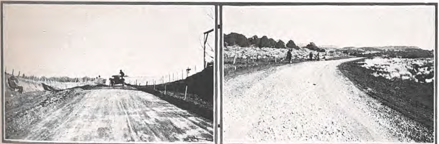
Showing method of constructing new federal aid crushed rock surfaced highway located east of Durango in La Plata county. Photo on left shows subgrade before application of crushed rock.
