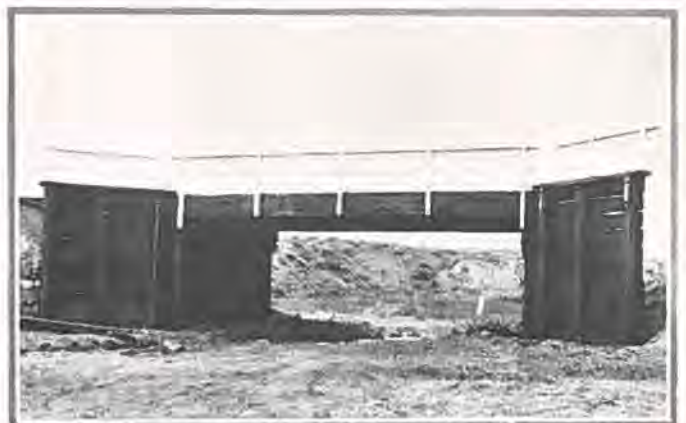
Type of creosote wooden bridge being constructed by the department on secondary roads.
