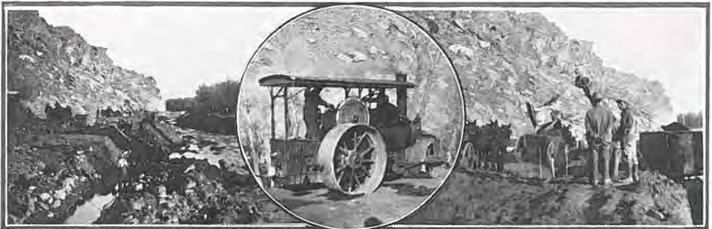
Showing construction crew taking a "kink" out of State Road No. 8 near the town of Morrison, preparatory to paving with cement concrete
