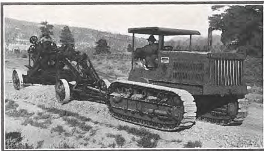
One of Colorado's heavy-duty maintenance outfits working on State Road No. 10, near Durango, in La Plata County.
