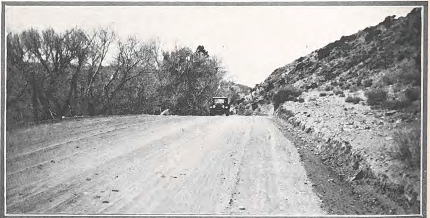
A beautiful stretch of state highway on the west slope of La Veta Pass, located in Costilla County, showing splendid condition resulting from efficient work of state maintenance crew. Photo by Patrolman Cummings.
