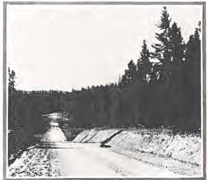
View of new Willow Creek Pass highway, which is being improved by the U. S. Bureau of Roads.
